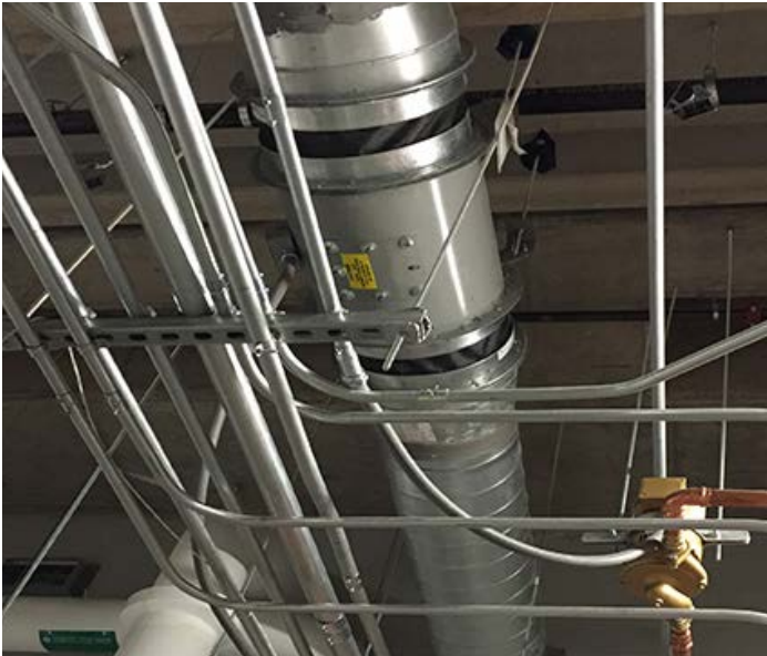
The water heater combustion SFTA air supply fan
